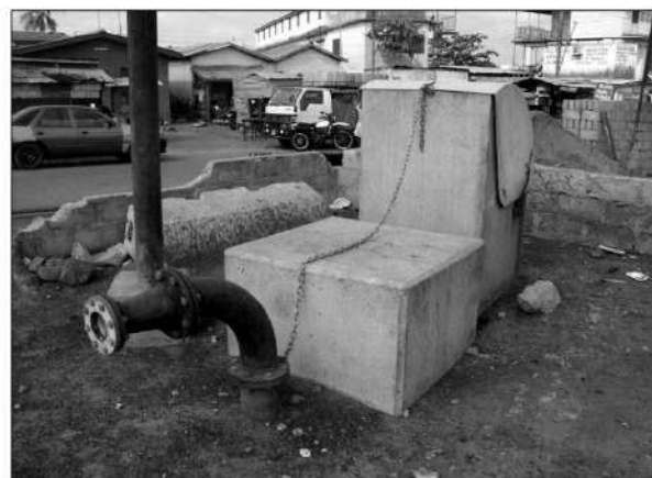
Top of an underground holding tank, showing a chain to lock the lid, a vent pipe and a wall to prevent overflowing excreta travelling onto the road! Source: Boot, 2008
